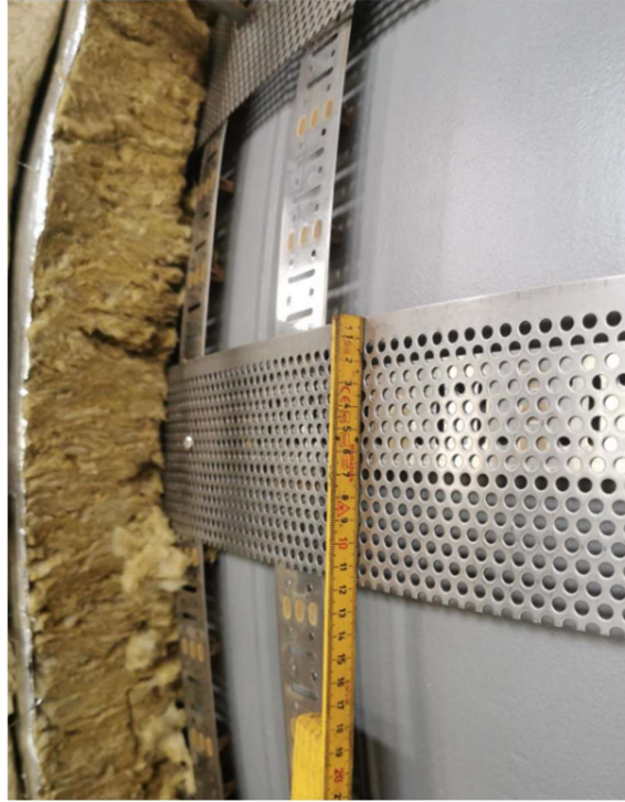
Figure 3: ESSGE NCS band on a large tank with maximum 400mm spacing
